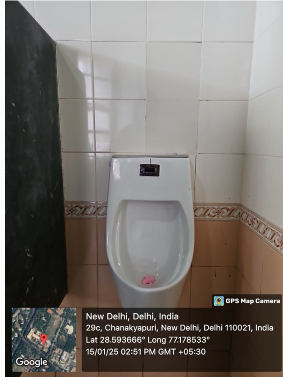
ADVANCED SENSOR BASED TOILETS TO REDUCE WATER CONSUMPTION IN WASHROOMS
